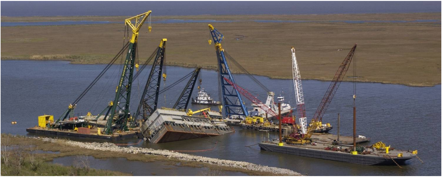
T&T Bisso refloats the inland drill barge using four derrick barges and a pull barge.
