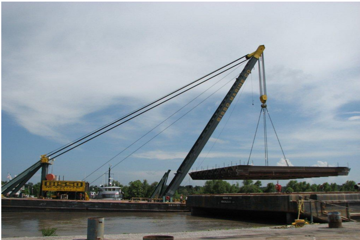
The D/B CAPPY BISSO lifts a 275-ton section of a subsea basket onto a materials barge in Belle Chasse, La.
