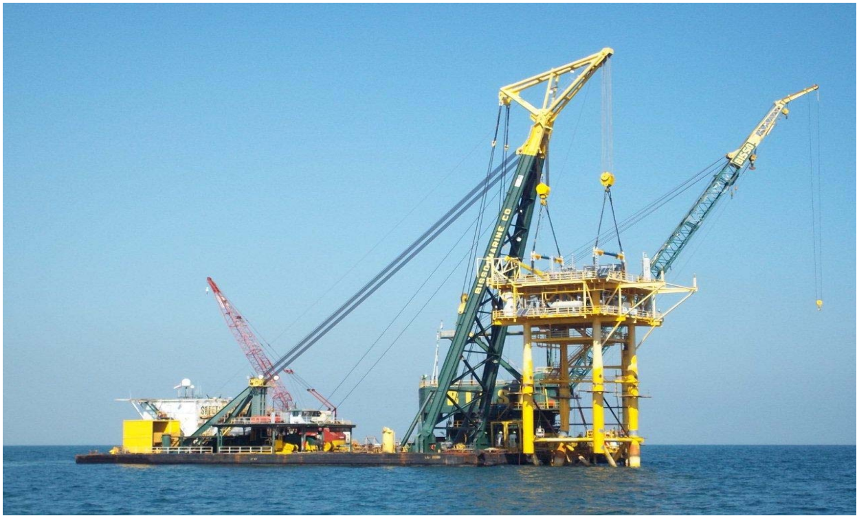
BISSO MARINE used the D/B LILI BISSO to perform a tandem block lift of an offshore production topside.
