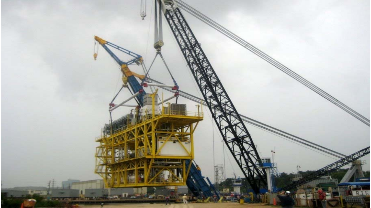
The D/B BIG-T and the D/B BIG JOHN perform a tandem lift of two 690-ton offshore modules.
